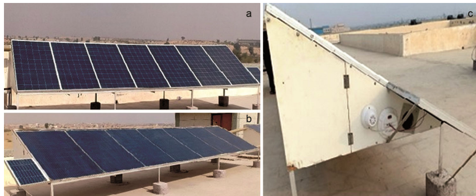
Fig. 1 — Installed experimental setup, (A) opaque PVT Array, (B) semi-transparent PVT Array and (C) Inlet side view.
