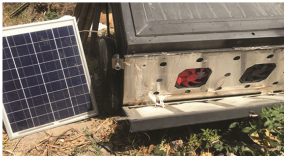
Fig. 3 — Two DC fans powered by a solar panel
